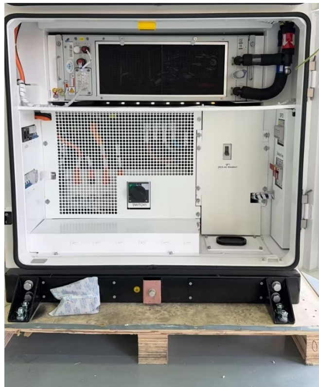
Picture 8 Electrical cabinet
