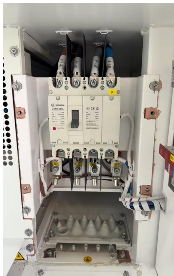
Picture 10 AC main circuit breaker
