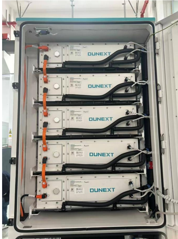
Picture 7 Battery cabinet
