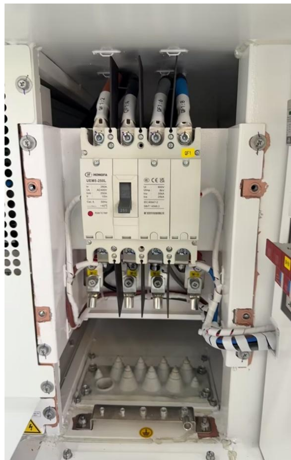
Picture 10 AC main circuit breaker
