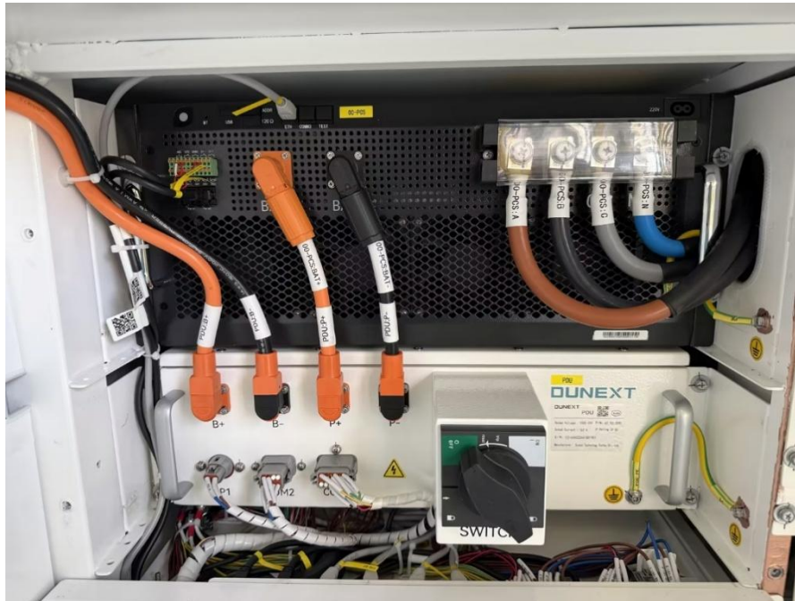
Picture 9 High voltage box/PDU + PCS box
