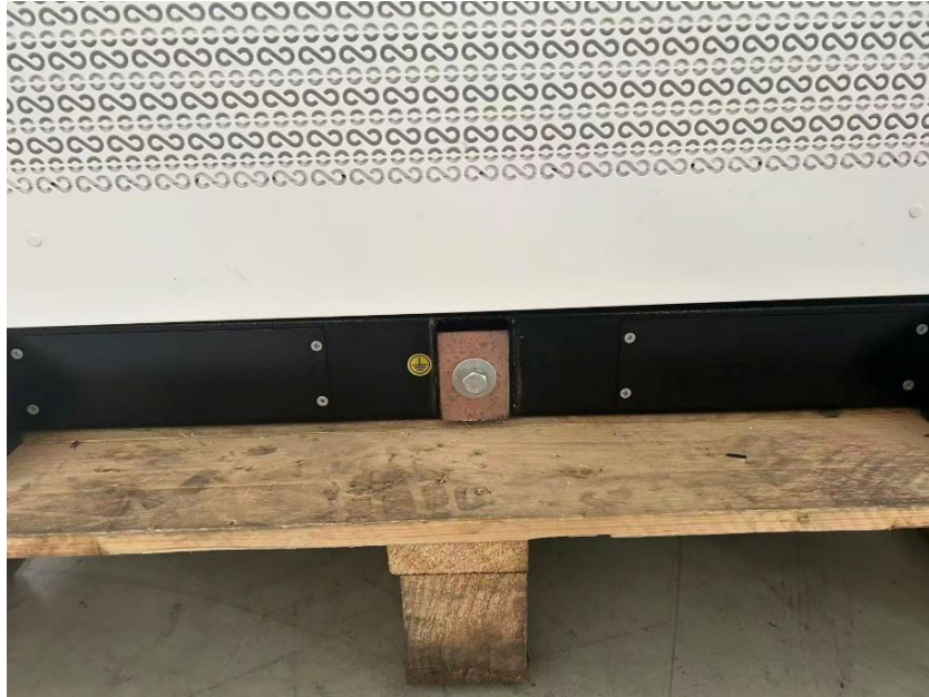
Picture 11 Earth terminal
