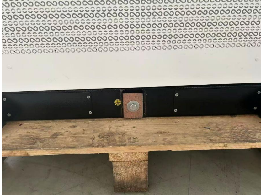
Picture 11 Earth terminal
