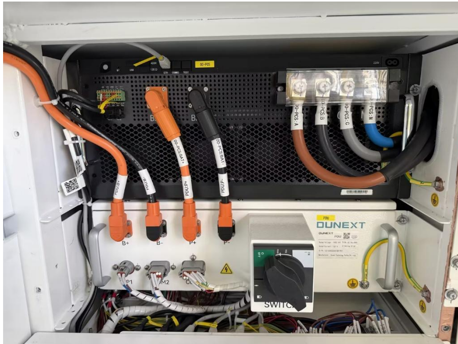
Picture 9 High voltage box/PDU + PCS box
