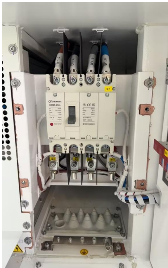
Picture 10 AC main circuit breaker
