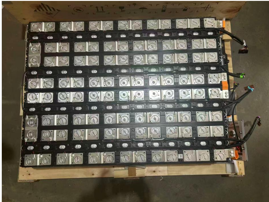
Picture 15 Battery pack (Inside view 1)
