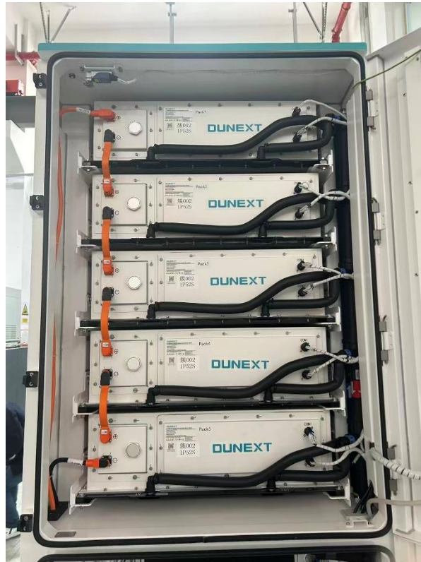
Picture 7 Battery cabinet
