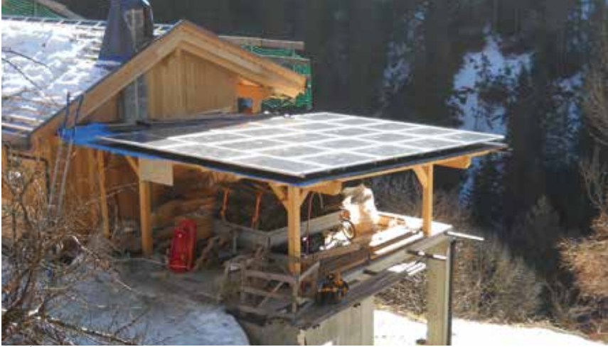
Elpo | St Vigil Enneberg - Italy System: 5.29 kW | Hanger Bolt System
