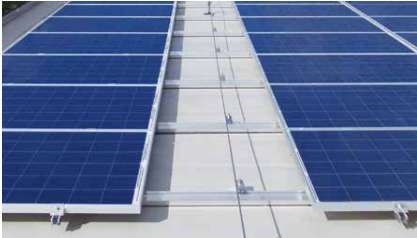
Elpo | Frubona Terlan - Italy System: 671.86 kW | Hanger Bolt System
